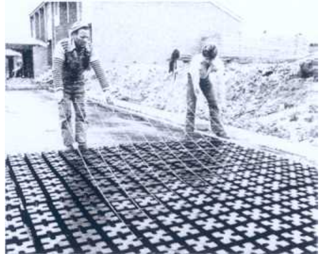
Polystyrene formers set up ready for pouring, showing steel reinforcing mesh being positioned.
